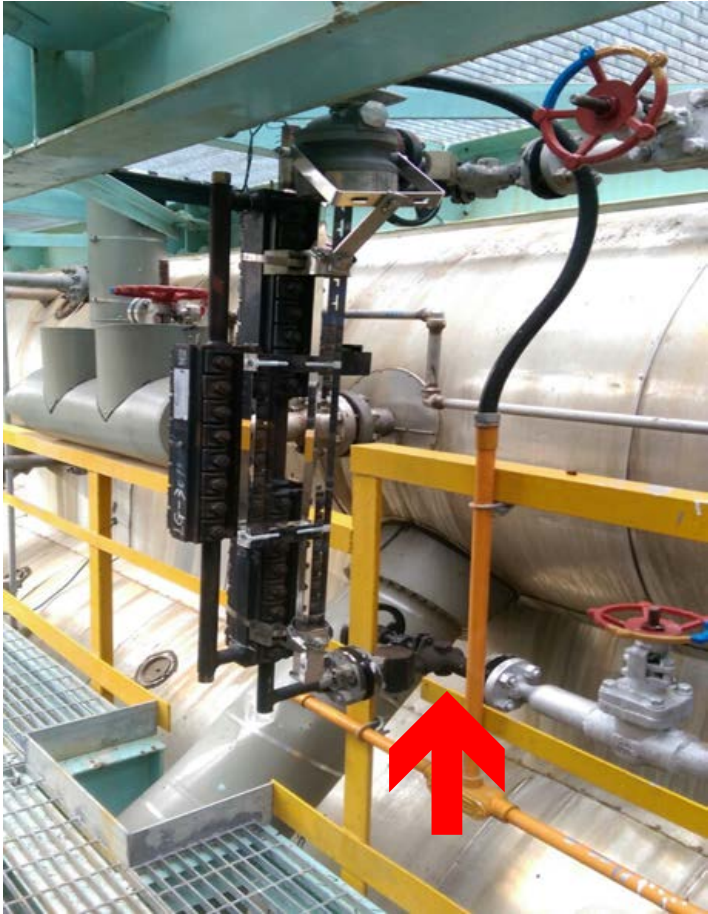
A drain valve is missing on this lower water gage valve
