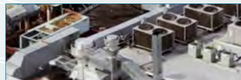
High performance HVAC controls
