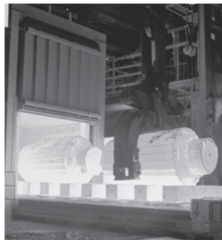
Butterfly valve BVHM on forging furnace to reduce the oxygen level
